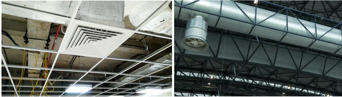
Exposed Metal Ducts
